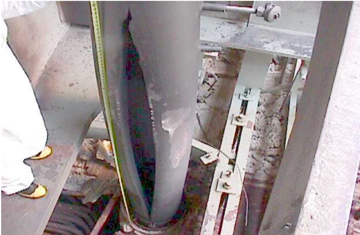
Figure 2. Photograph of seam-welded pipe failure at Hawthorn Unit 5.
