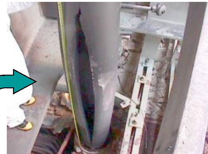
August '98 failure of Hawthorne 5 SH link piping. This was the 2nd catastrophic failure of SH link piping in two years (Mt. Storm Unit 1 in June 1996). The piping was not known to be seam welded from supplied documentation.
